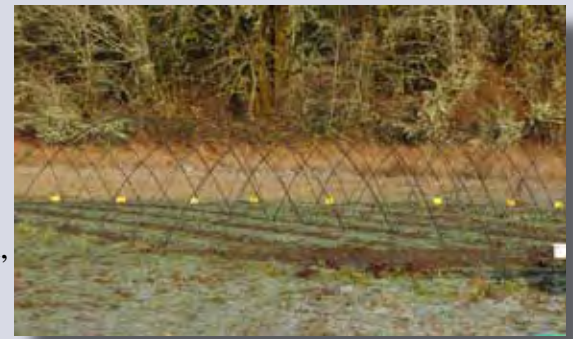
An experimental hoophouse design using rebar lined with used drip tape, promising but untested at Gales Meadow Farm. Photo by Nick Andrews
