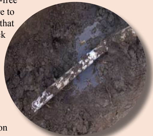
An unprotected pipe broken by winter temperatures. Photo from Wiki Commons
